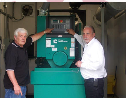
Steve Svetkovich, Maintenance Supervisor, Sisters of Charity of Seton Hill, and Bill Castile present the generator for the new water pumping station.
