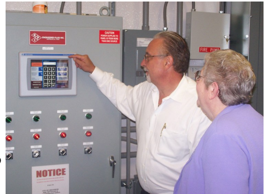
Bill Castile, water distribution facilities Superintendent, Municipal Authority of Westmoreland County shows Sister Vivien Linkhauer, Provincial Superior, Sisters of Charity of Seton Hill, the control center for the new water pumping station located at the bottom of Mount Thor Road.
