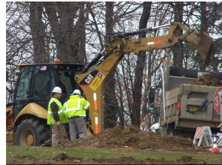
Crews broke ground on Monday, March 15, 2010 near the entrance to the employee driveway at Caritas Christi.
