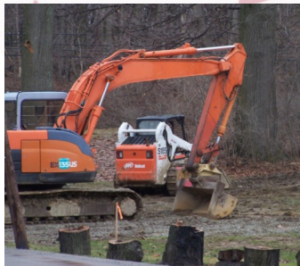
Equipment is in place to begin construction at the bottom of Mount Thor Road.
